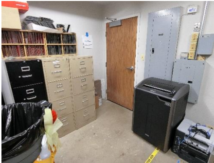
Records storage in mechanical room
