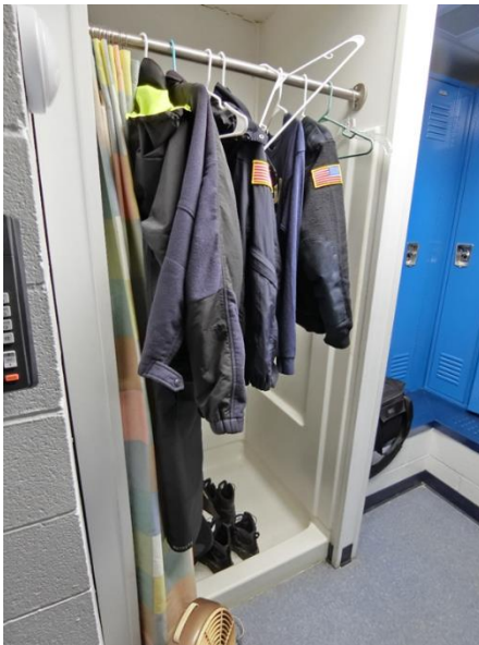
Women's locker room shower used for storage
