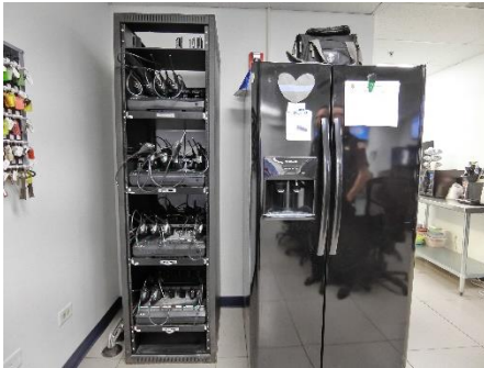
Patrol office radio charging and refrigerator area
