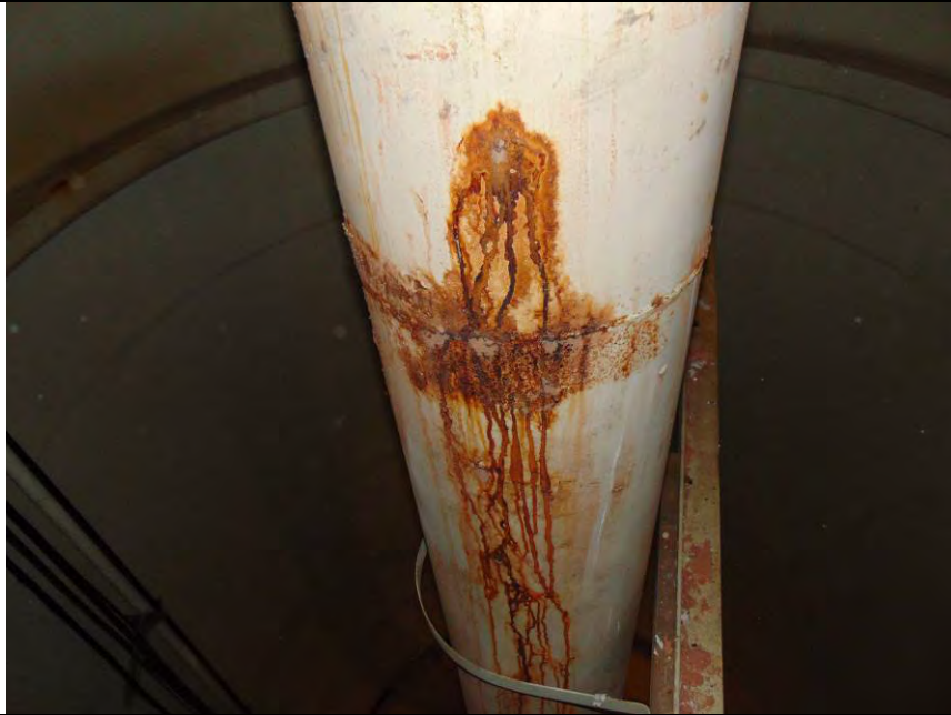
Photo 6 Leak at approximately 60' above the condensate platform.
