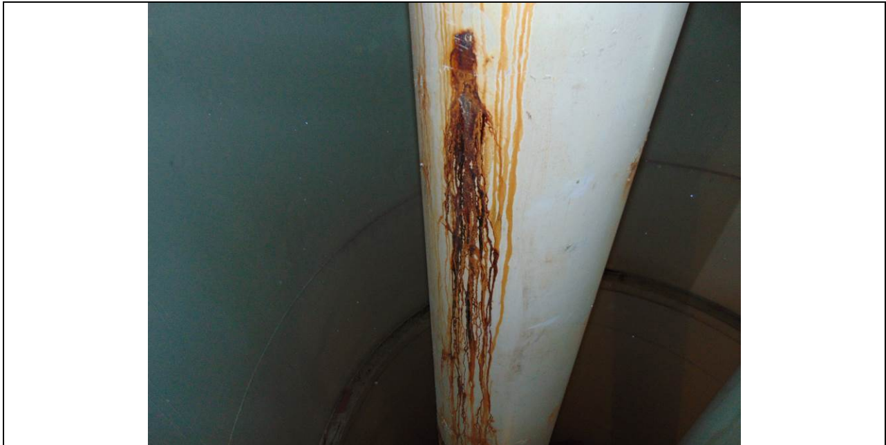
Photo 4 Leak at approximately 30' above the condensate platform.
