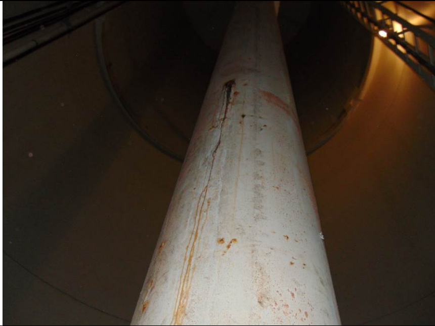
Photo 8 Possible leak at approximately 70' above the condensate platform.
