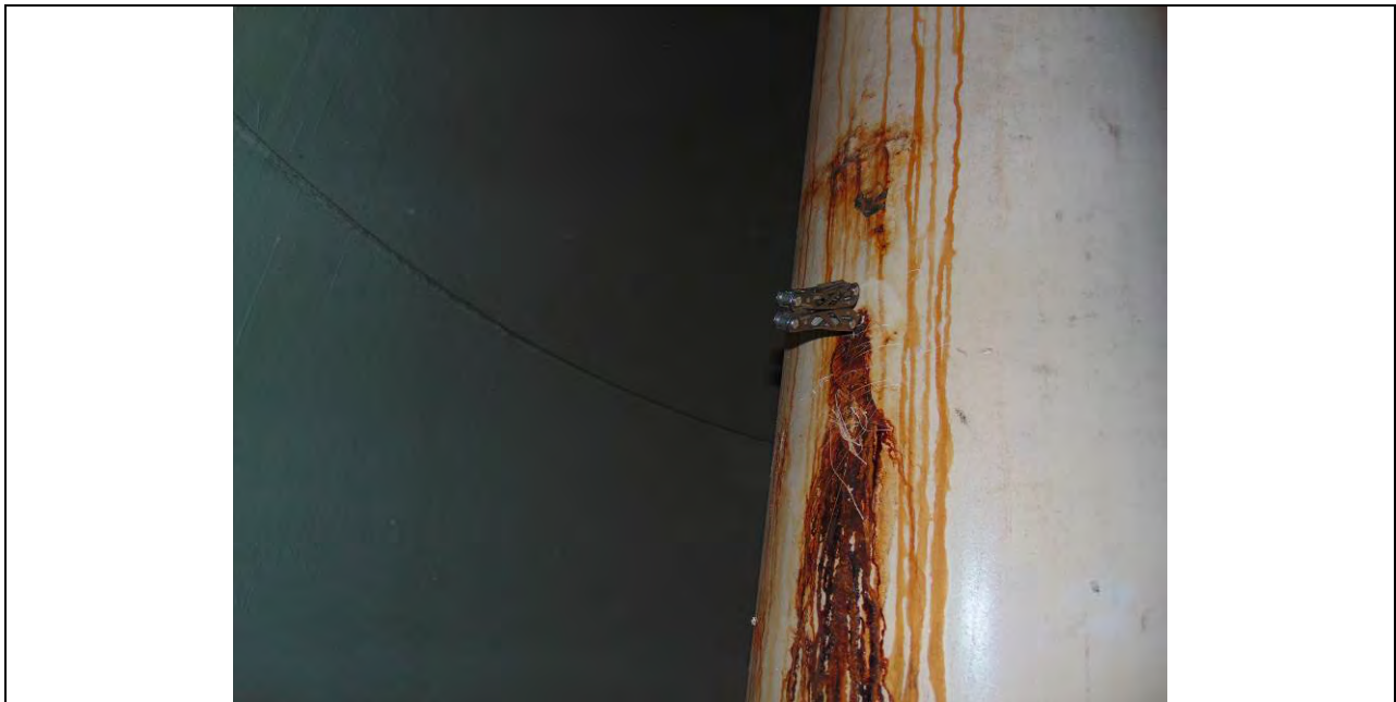
Photo 5 Leak at approximately 30' above the condensate platform.
