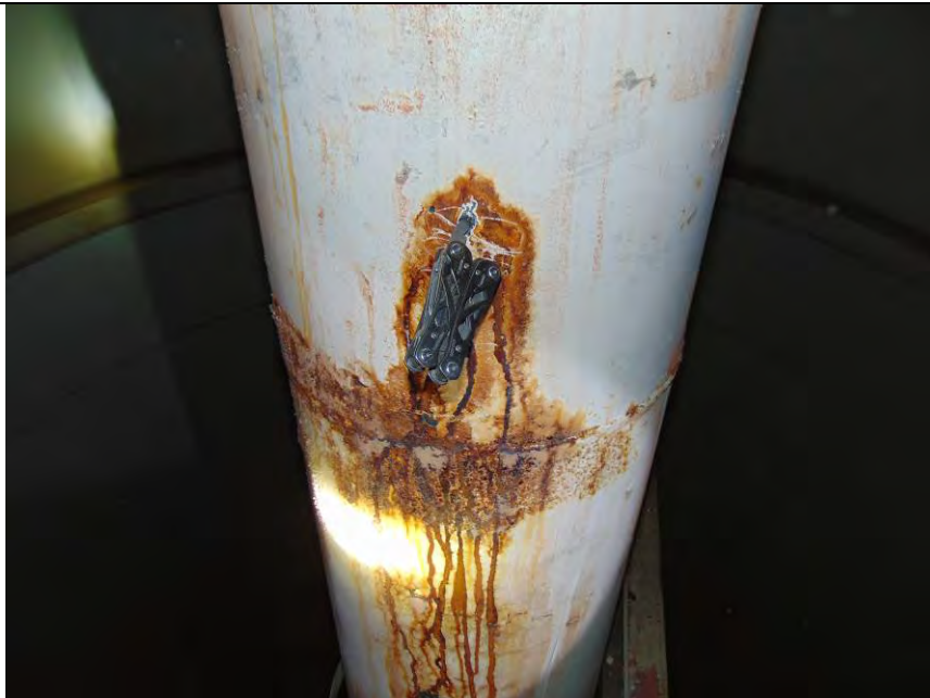
Photo 7 Leak at approximately 60' above the condensate platform.
